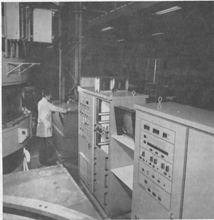
Figure 6 : View of the control panel of the equipment.
